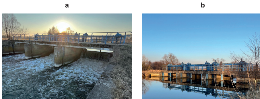
Fig. 3. The damming weir on the Radomka in Piaseczno: a – downstream view, b – upstream view of the structure with the impounded water level
