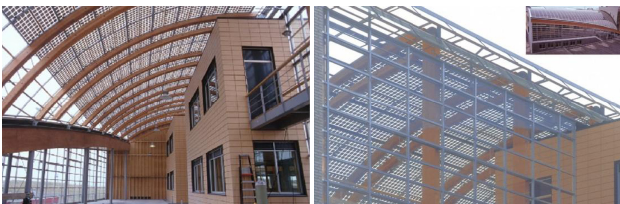
Fig. 4. Glazed BIPV as a covering for a winter garden in the ECN-42 office building in Petten, the Netherlands
