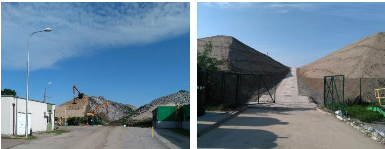
Fig. 4. Landfill during the construction of the layer separating the waste from the subsequent reclamation layers (left) and the final result (right) – view of the landfill entrance
