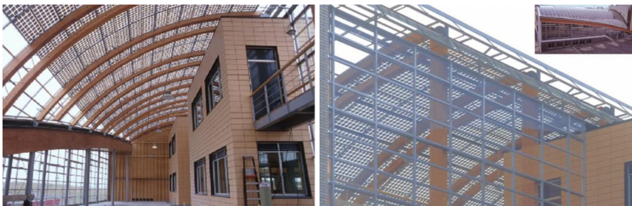
Fig. 4. Glazed BIPV as a covering for a winter garden in the ECN-42 office building in Petten, the Netherlands
