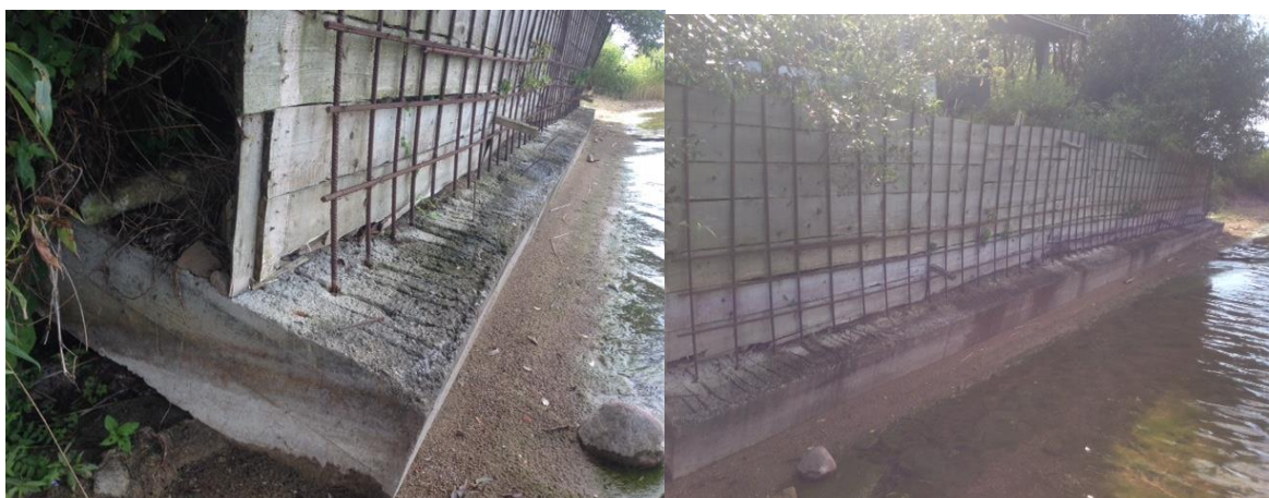
Fig. 2. The deformations and deteriorations of existing reinforced concrete retaining wall
